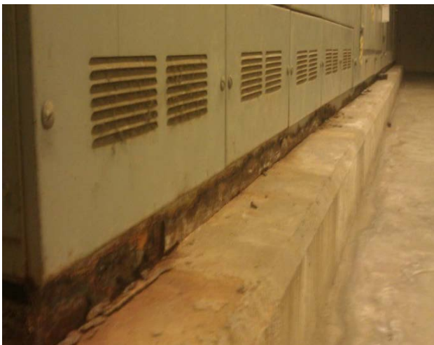
Current Condition of the Founders Hall Switchgear
