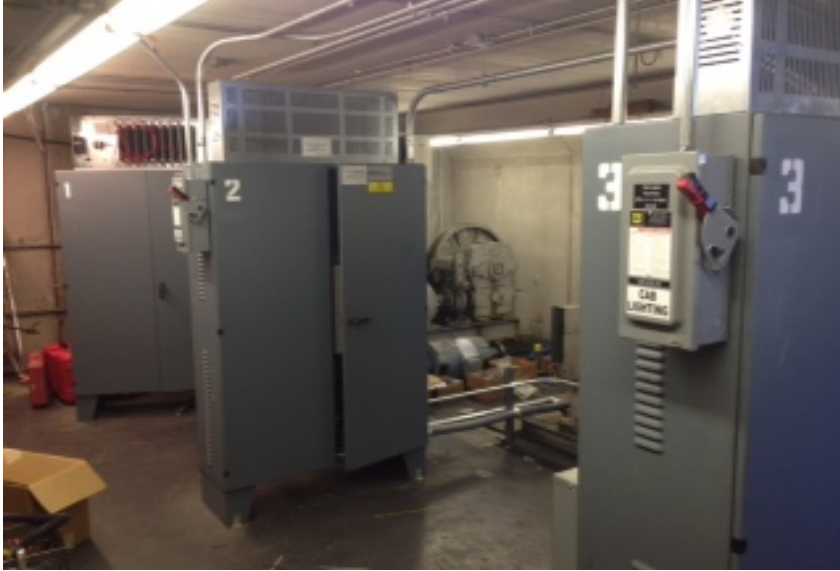
Landrum's New Elevator Control Equipment
