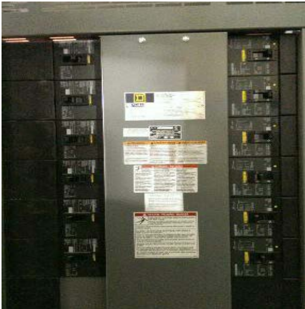
Electrical Equipment with Installed Safety Labels.
