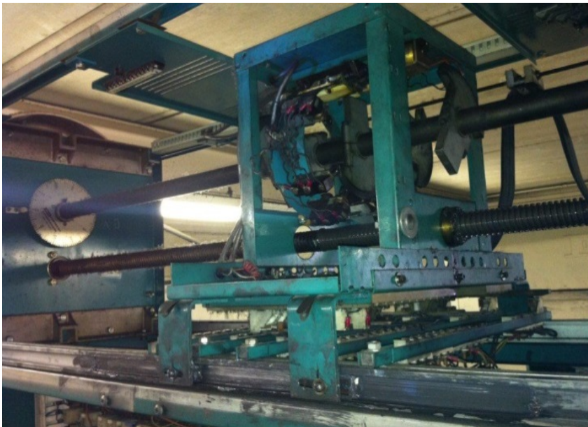
Landrum's Old Elevator Control Equipment
