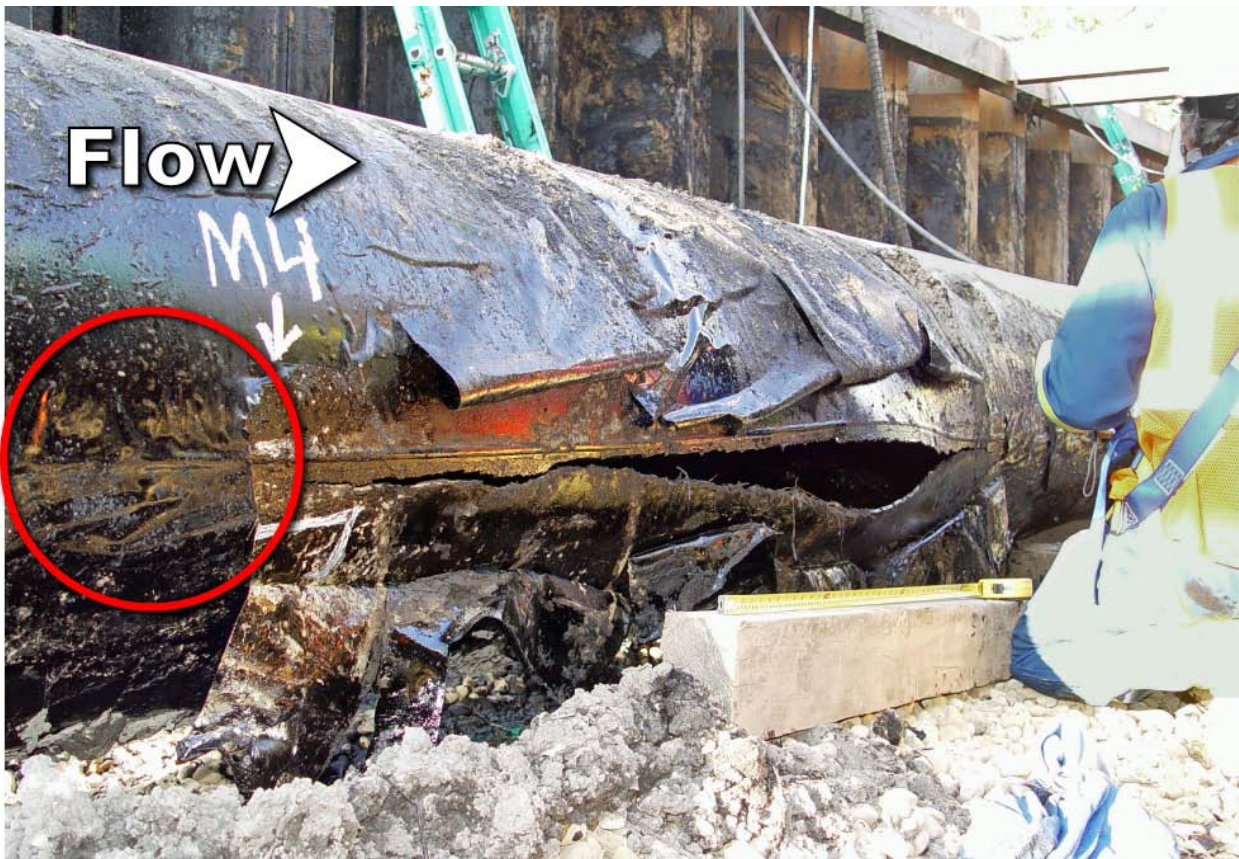
Figure 2. The ruptured segment of Line 6B in the trench following the July 25, 2010, rupture. The fracture face measured about 6 feet 8.25 inches long and was 5.32 inches wide at the widest opening. The fracture ran just below the seam weld that was oriented just below the 3 o'clock position. A red circle shows a location where the coating was wrinkled and had separated from the pipe surface.
